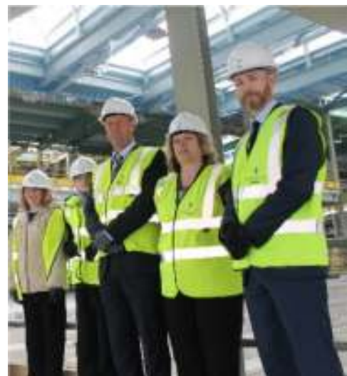
Viewing the shell of the new build Mr P. Thomas, Mrs C. Edwards and pupils with a member of Willmott Dixon Construction
